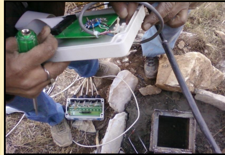
Piezometer connection to JCB
