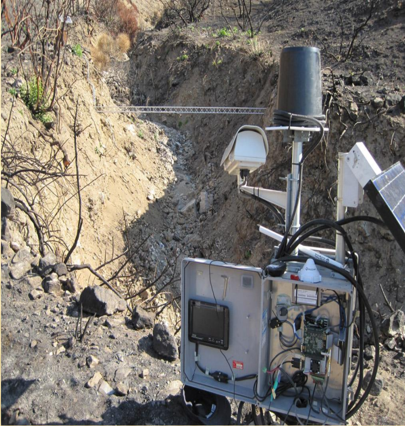
Video Monitoring System
