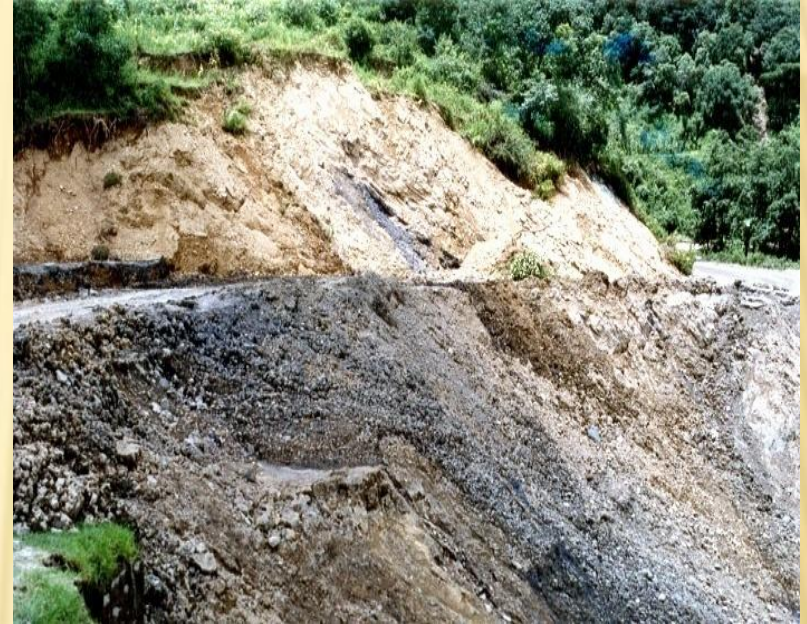
9 th Mile Landslide on NH - 39
