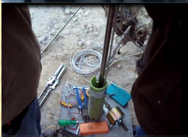
Lowering of Sensor
