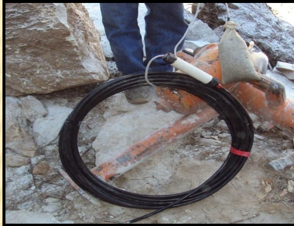
Piezometer secured in Sand Bag
