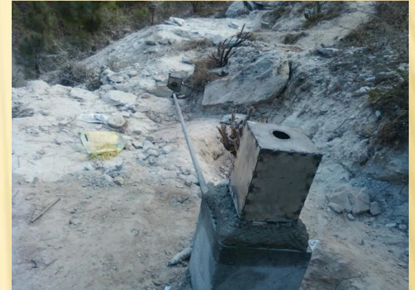
IPI wires to JCB within GI Pipe
