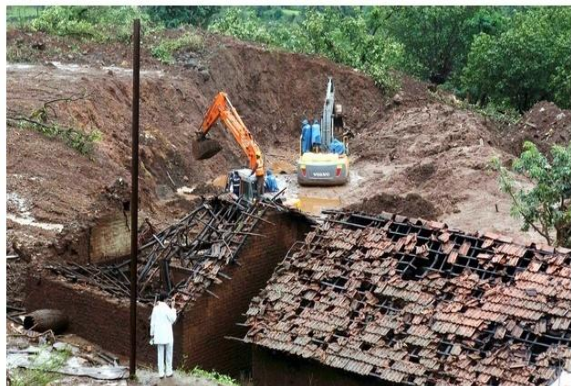
Rescuers search for survivors among the debris of houses at landslide-hit Malin village in Pune Maharashtra on Friday | PTI Photo
