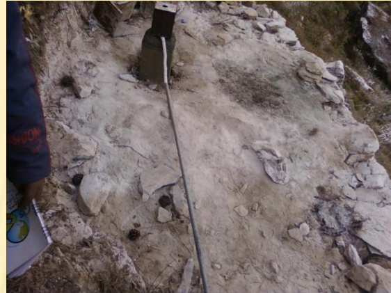
IPI wires inside GI Pipe
