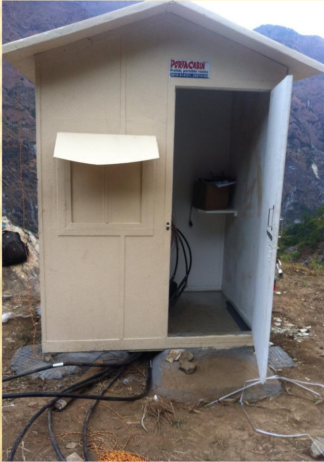
CONTROL STATION (HUT) TO HOUSE INSTRUMENTS
